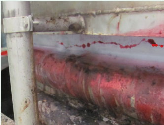
Crack in vessel wall (visible with red die)
