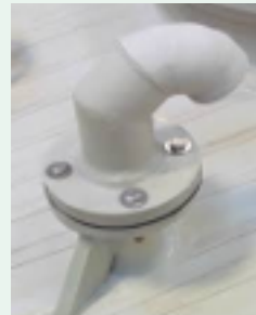
A larger vent size was installed after the incident
